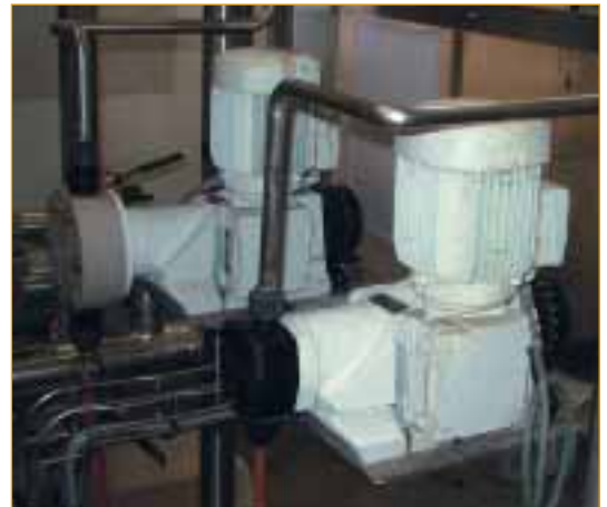
Metering of soda and acid
